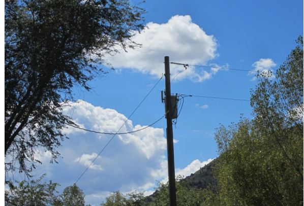
PHOTOGRAPH NO. 14 View of pole mounted transformer on north adjacent site looking west
