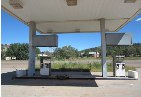
PHOTOGRAPH NO. 13 View of pumps and canopy looking east
