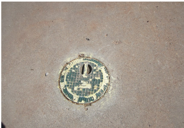
PHOTOGRAPH No. 11 View of diesel fill port
