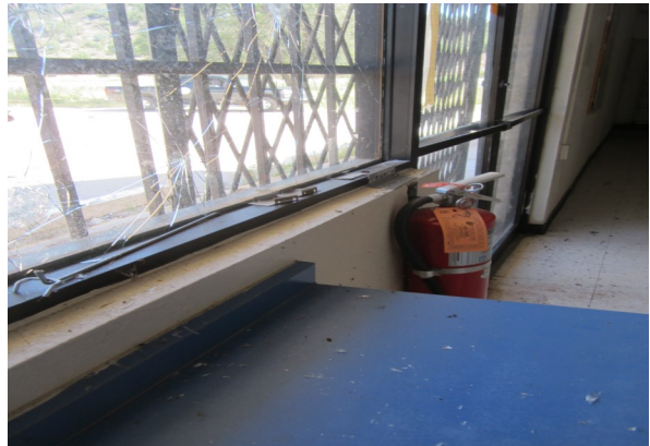
PHOTOGRAPH NO. 8 View of inside of convenience store looking at the fire extinguisher
