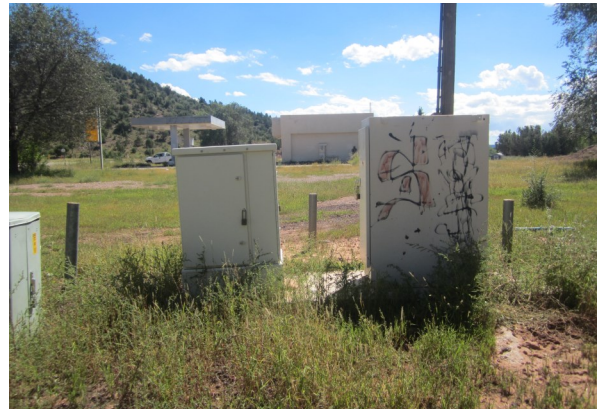
PHOTOGRAPH NO. 16 View of transformers on north adjacent site looking south
