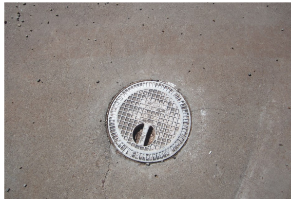
PHOTOGRAPH No. 12 View of unleaded fill port
